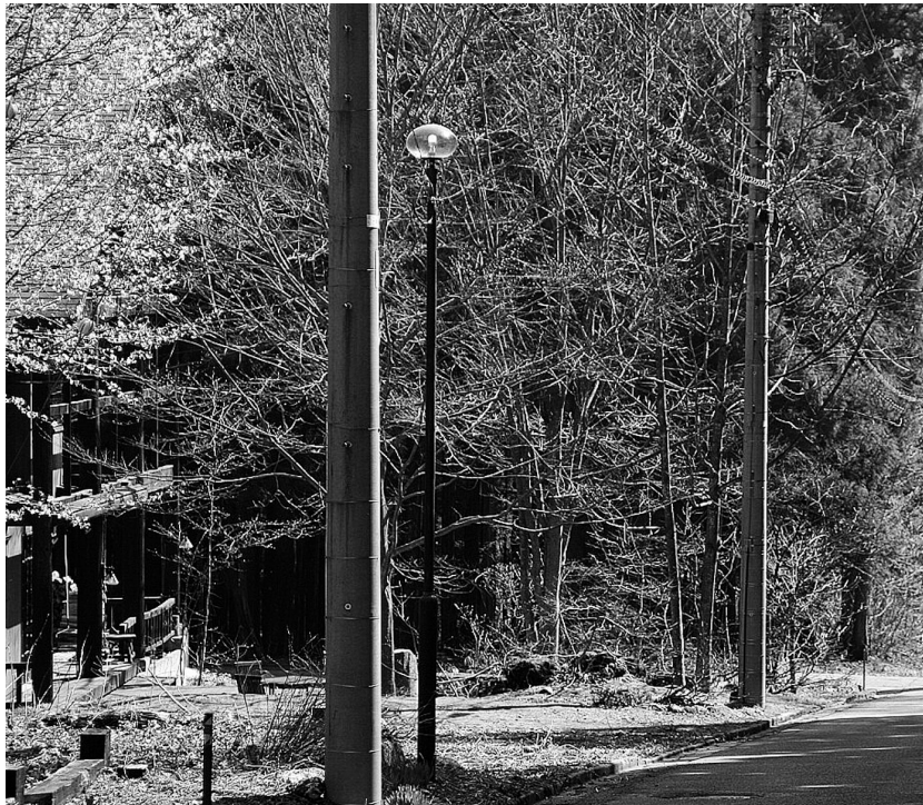
LED化が進む街路灯
